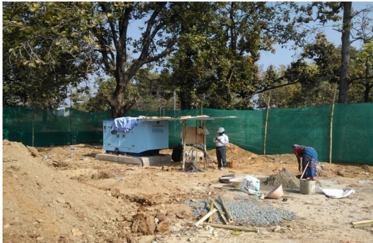
30 KVA DG SET INSTALLED
